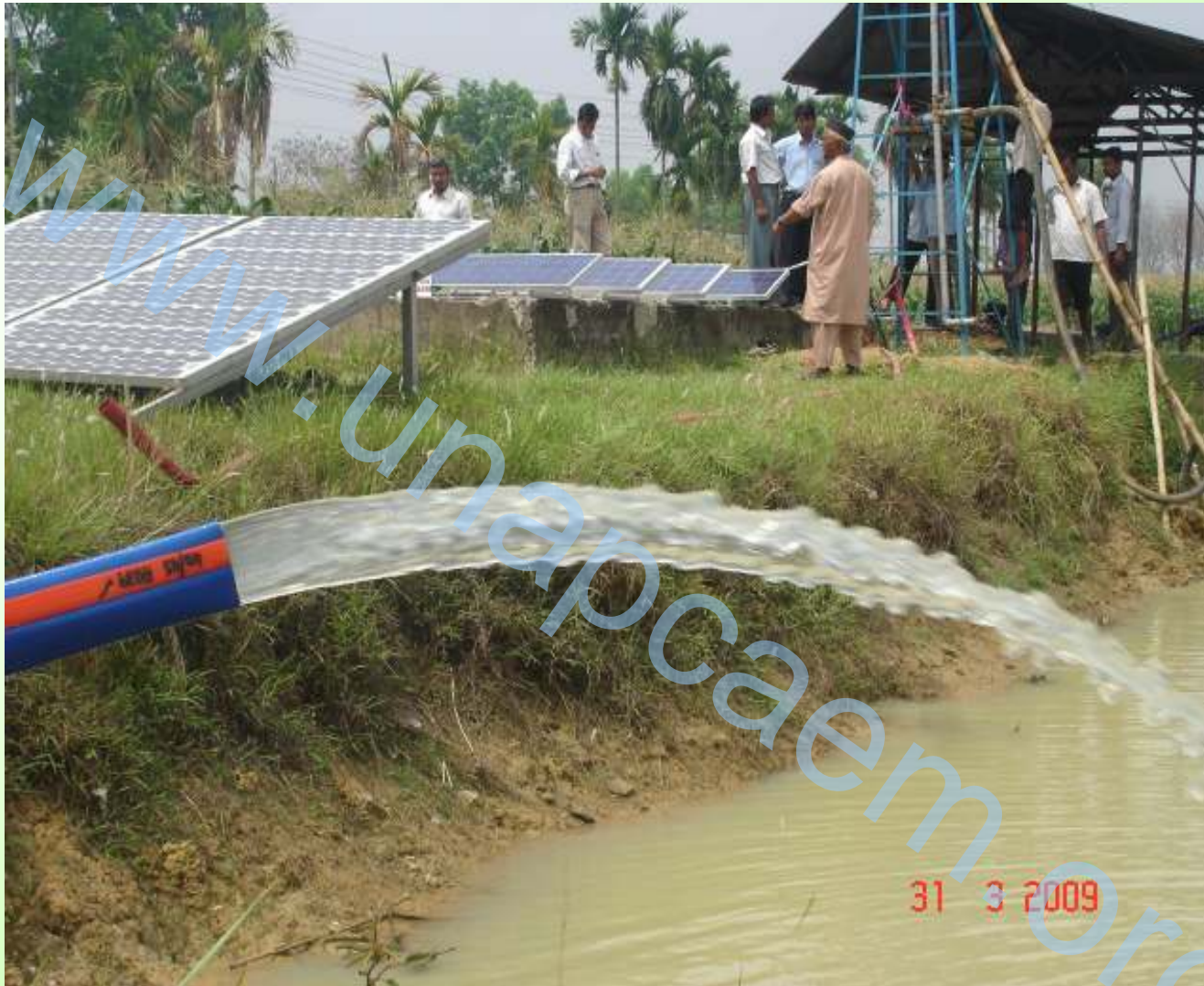
Discharge of Rahimafrooz owned solar pump
