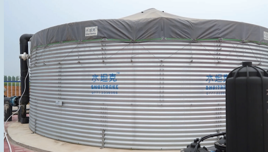
The water treatment device Water Tank
